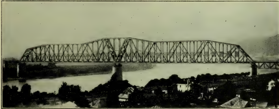
FIG. 6B.—Sciotoville Continuous Girder Bridge across the Ohio River, Two Spans of 775 Feet Each
